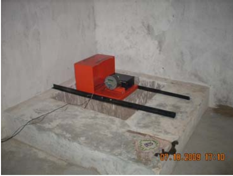
Digital Water Level Recorder installed at Kanpur (UP)
