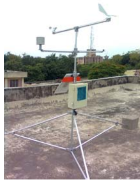
Automatic Weather Station Installed at Allahabad (India)
