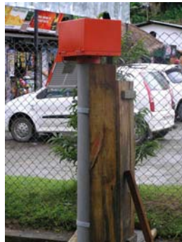
Automatic Water level Recorder installed at Nongpoh, Meghalaya, India
