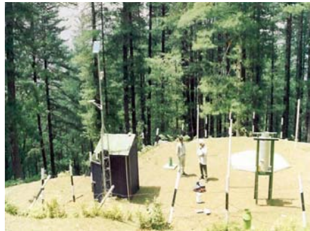
Weather Monitoring System installed at CWC, J&K, India
