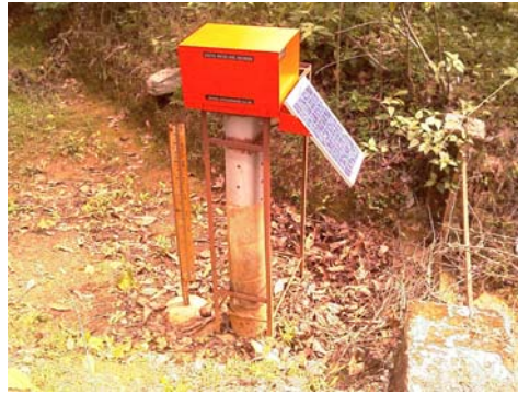
Digital water Level Recorder installed at Sirsi (Karnataka)
