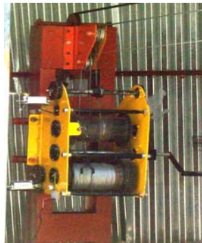
G&D Site installed at Holi (Himachal Pradesh), India
