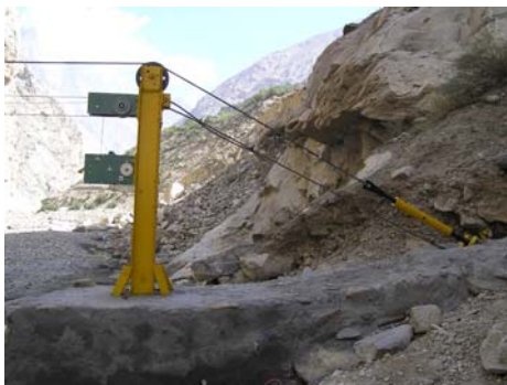
G&D Site installed at Khab (Himachal Pradesh), India
