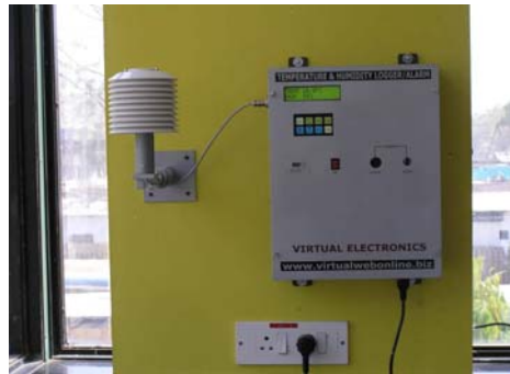
Air Temperature & Humidity Alarm System installed at , Kolkata
